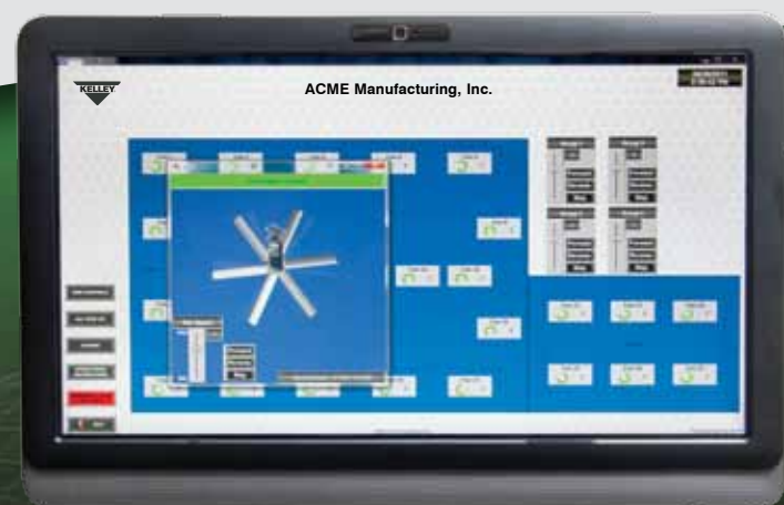
Dialog box for individual fan provides access to direction and speed settings for a specific fan.
